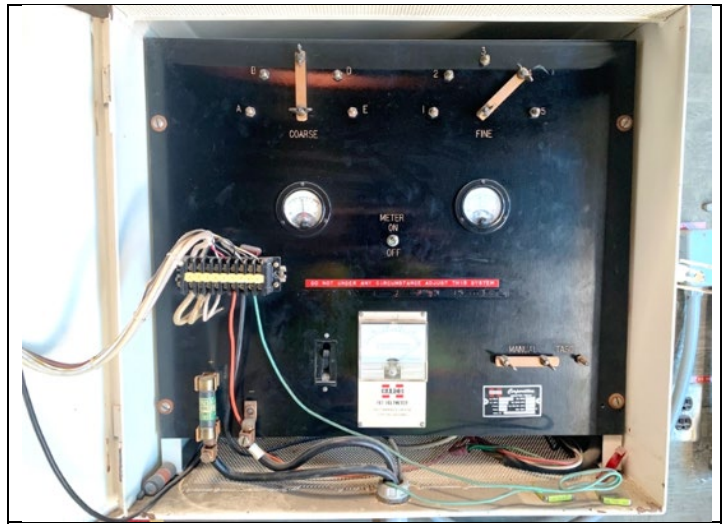
Photo: Impressed Current Rectifier
