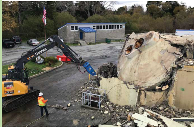
CAWD's circa-1930s digester was demolished in January to make way for new construction. We were able to get an amazing 85 years of service from the structure by converting it to a sludge holding tank after it had outlived its useful life.
