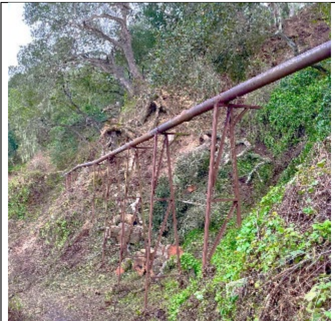
Photo: Aerial gravity pipe in easement
