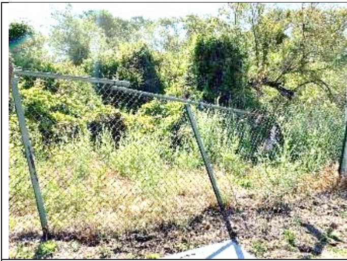
Photo: Existing dilapidated fence
