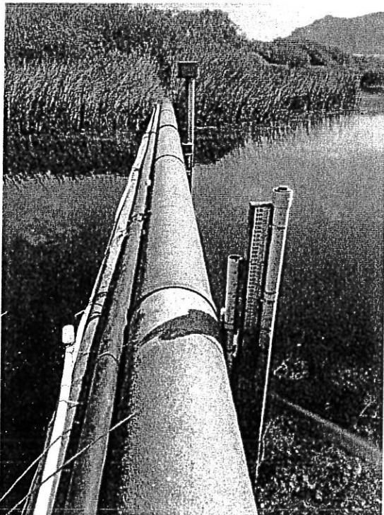
Photo 12: Top of pipeline. View looking east. Carmel River water level monitoring gauge near middle.
