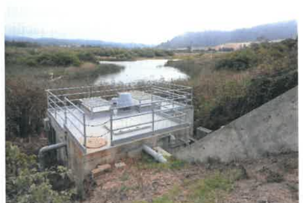
Calle la Cruz Pump Station
