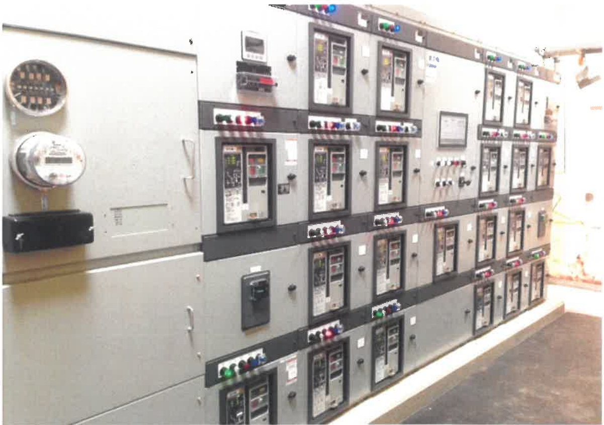
Primary Motor Control Center – installed 2017
