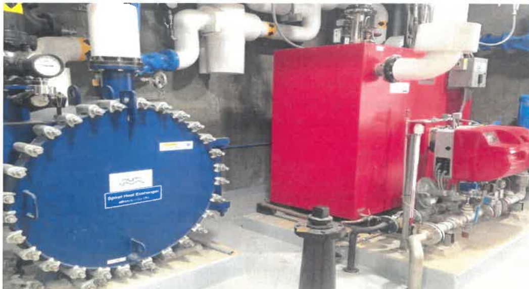
Digester Control Building #1 – Spiral Heater and Boiler
