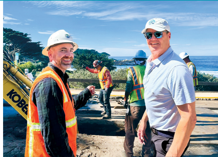
CAWD Engineer Patrick Treanor answers questions from Carmel resident Jim Messermer during construction near Jim's home on Scenic Drive.
