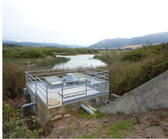
Calle la Cruz Pump Station
