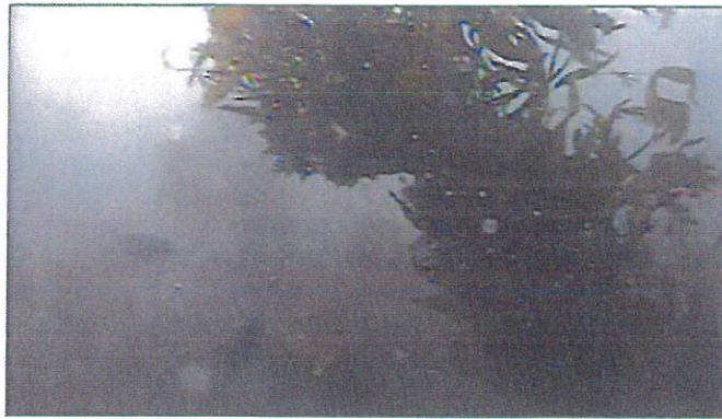
Figure 3 -- Overall view underwater of diffuser No. 4 showing the extent of kelp and marine growth. A rapid assessment of the diffuser is still possible, but finer detail is hidden by the growth.
