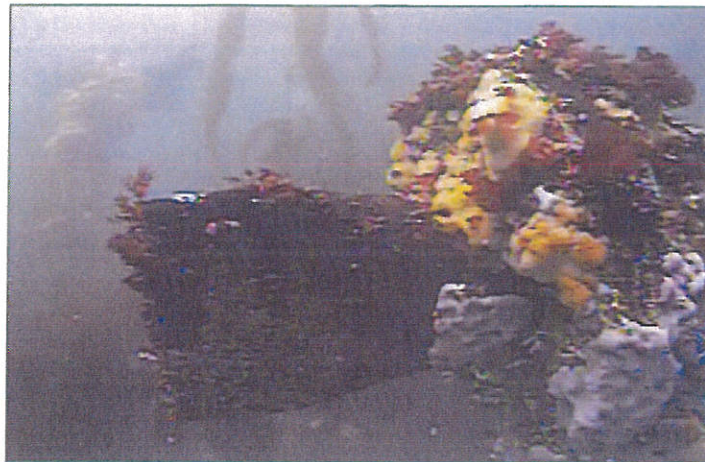
Figure 5 View underwater of a typical duckbill type backflow prevention valve and riser.
