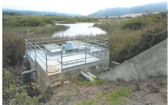
Calle la Cruz Pump Station
