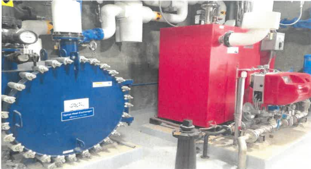
Digester Control Building #1 – Spiral Heater and Boiler
