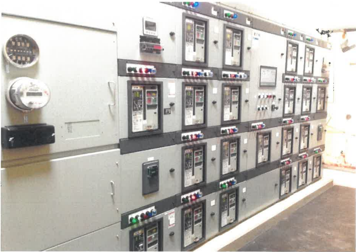
Primary Motor Control Center – installed 2017
