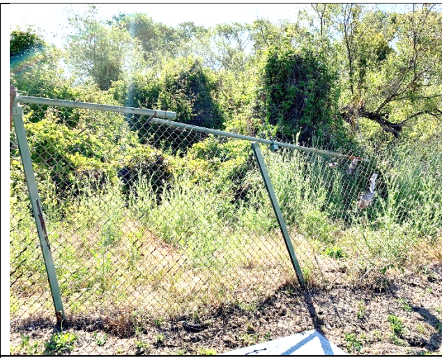
Photo: Existing Dilapidated Fence
