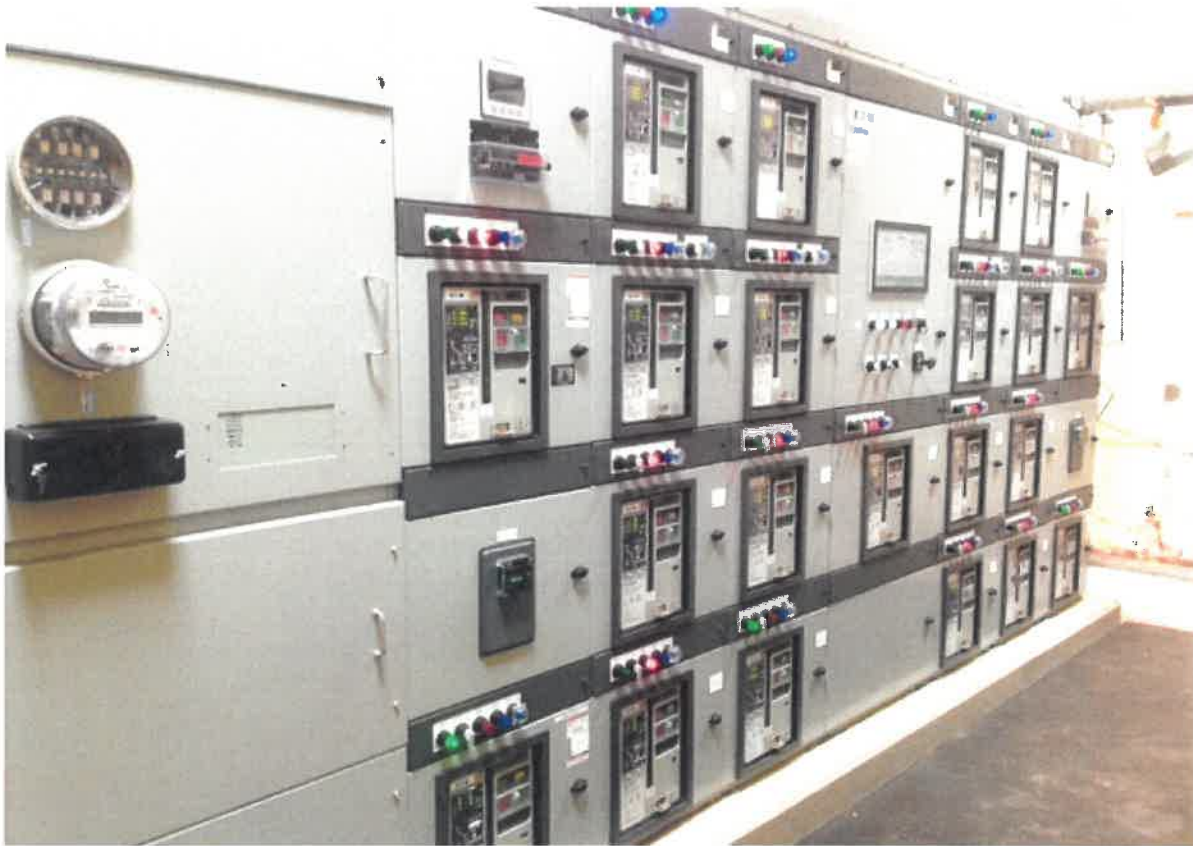
Primary Motor Control Center – installed 2017
