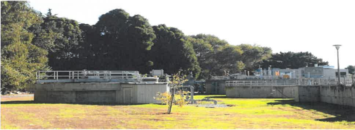
Clarifiers tanks & DAFT
