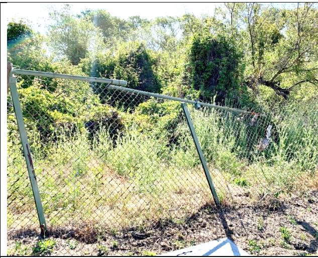
Photo: Existing Dilapidated Fence
