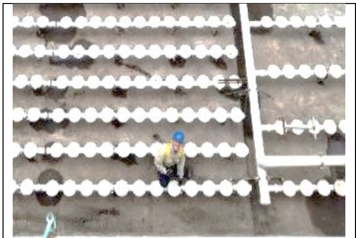
Photo: Existing air diffuser system
