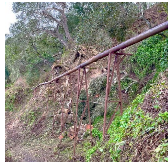
Photo: Aerial gravity pipe in easement
